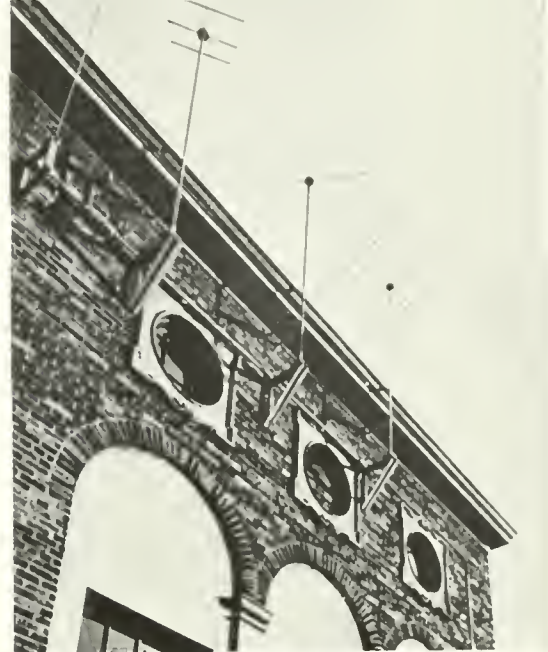
ANTENAPLEX INSTALLATION ON PARK LANE HOTEL IN NEW YORK.
